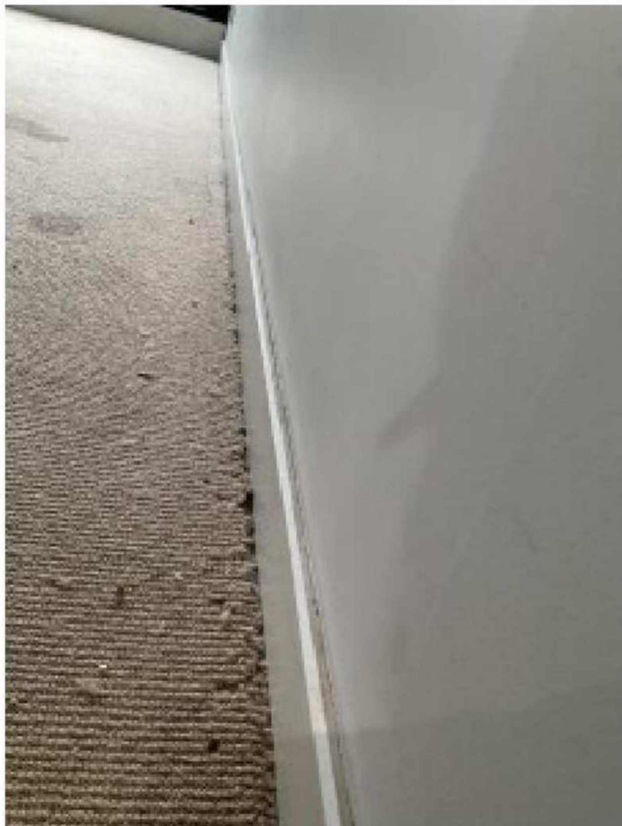
The carpet is shrinking away from the skirting. Consider consulting a professional for evaluation and potential corrective measures or replacement.
