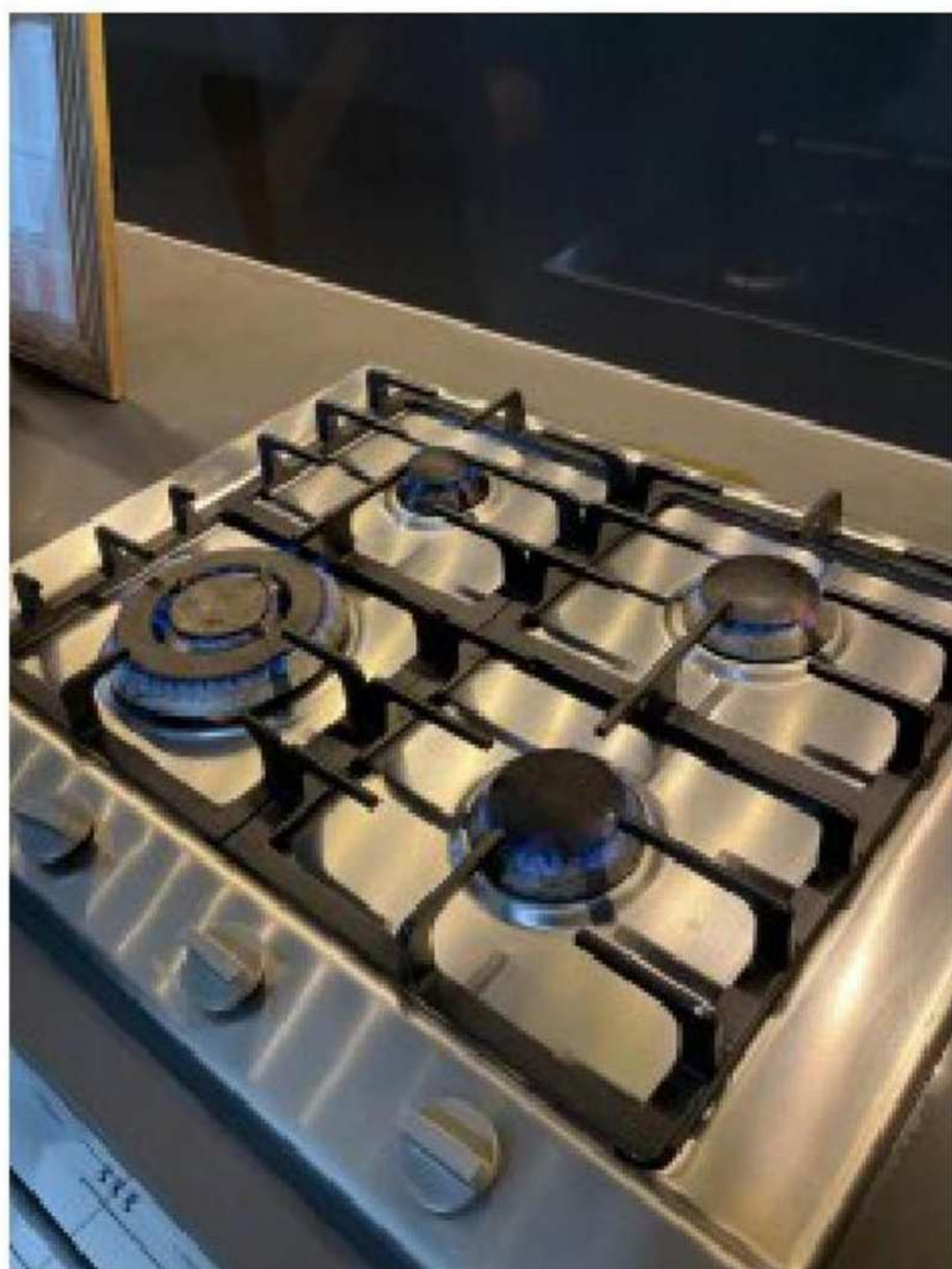
Cooktop is tested and operational at the time of inspection
