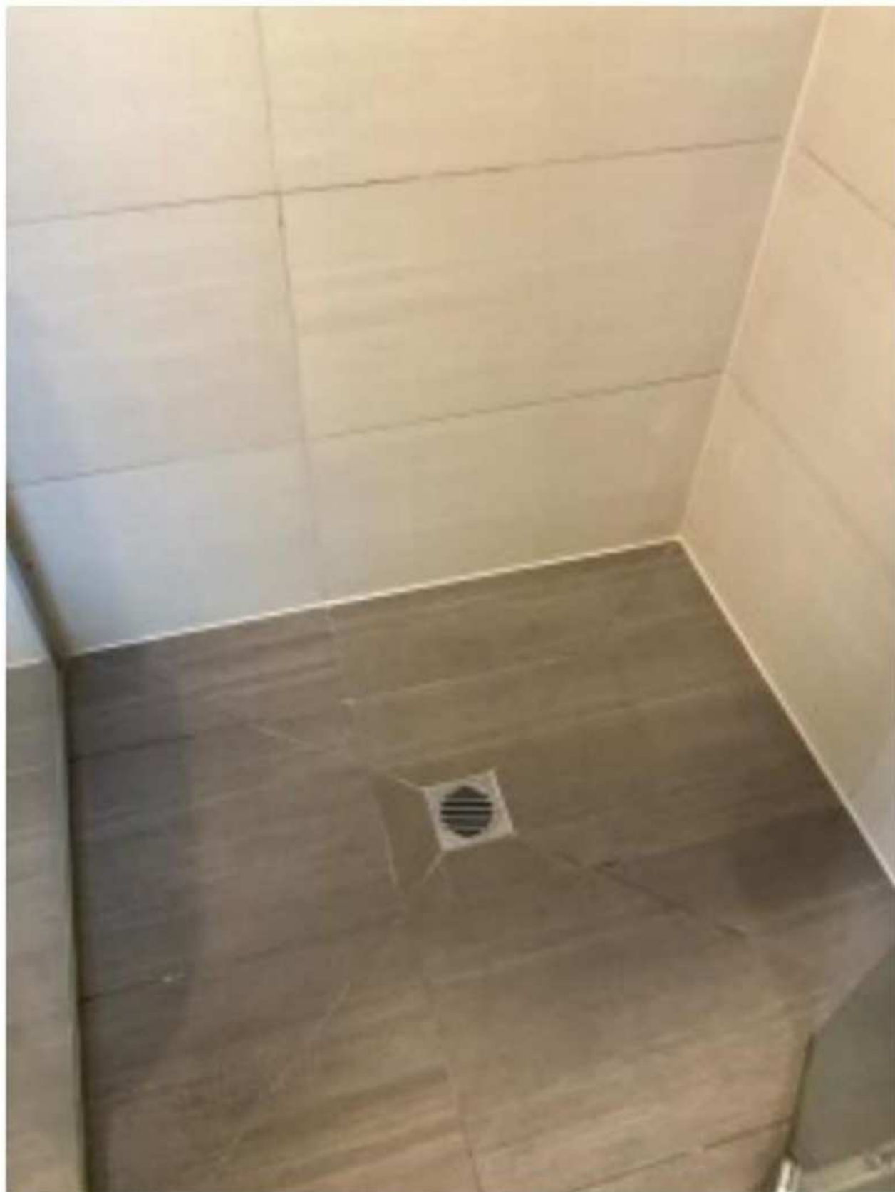
Visible signs of mould growth on the wall tiles and shower base in the bathroom. Recommend regular cleaning to prevent grout deterioration
