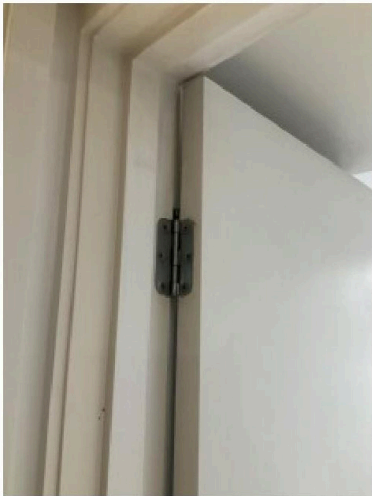
It appears the one of the door hinges pin is popping up from the fixing position. Recommended to fix the hinges to ensure smooth operation and proper alignment.
