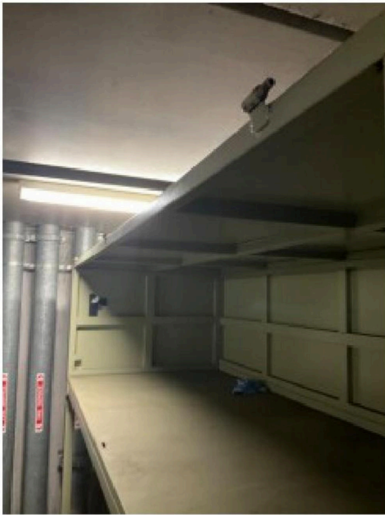
The storage room door in the car park is detached from its hinges. Recommended to repair the components and reattach and ensure it operates correctly and locks securely.
