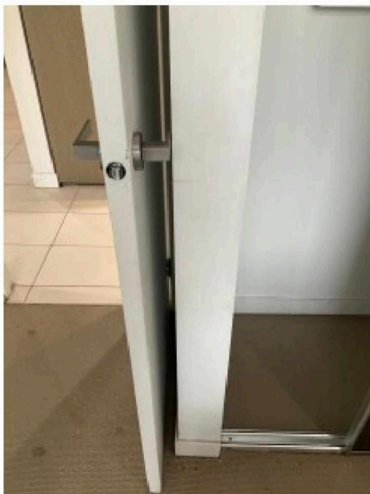
No door stop fitted at the time of inspection
