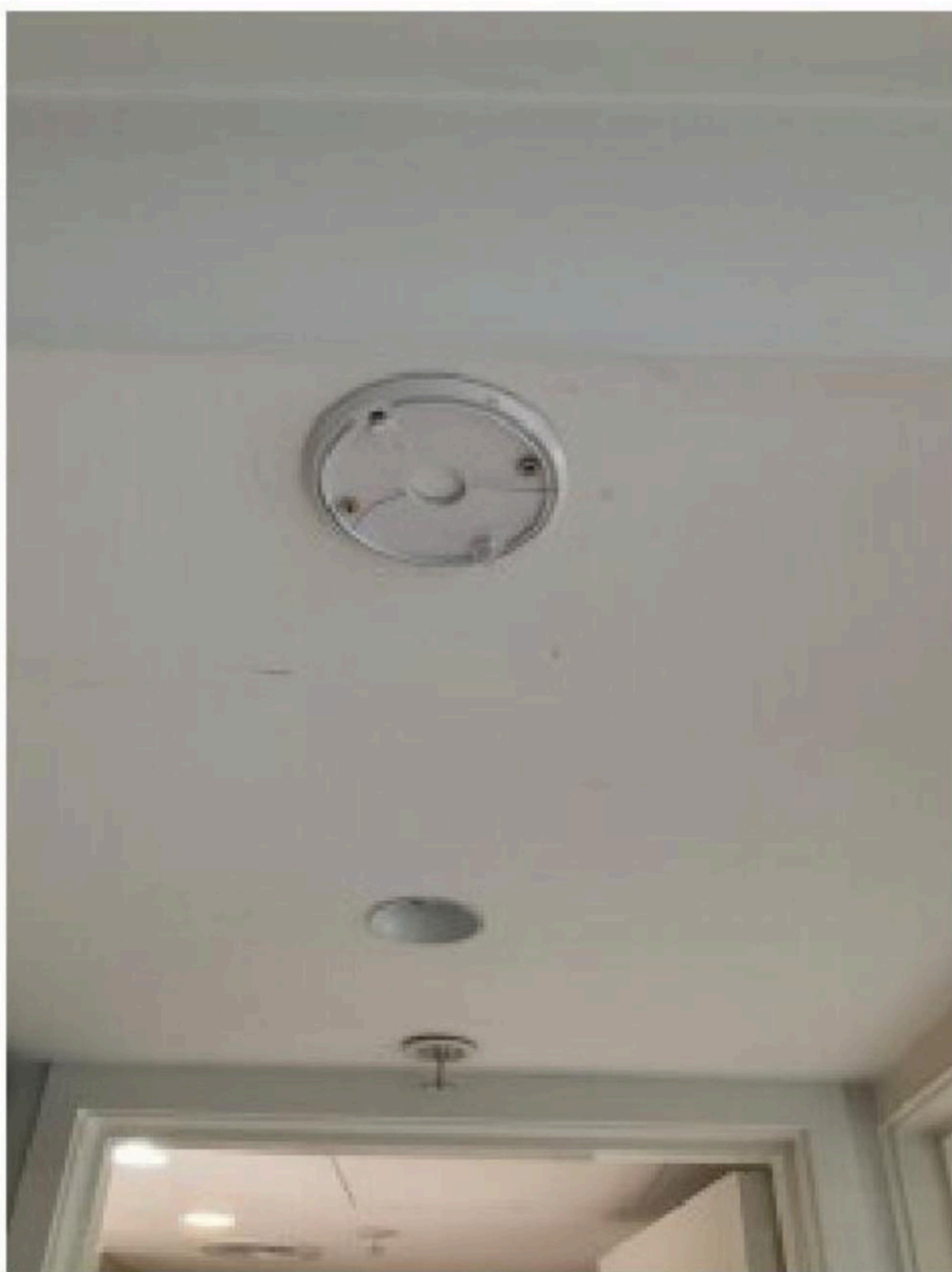
Smoke detector not in place at the time of inspection
