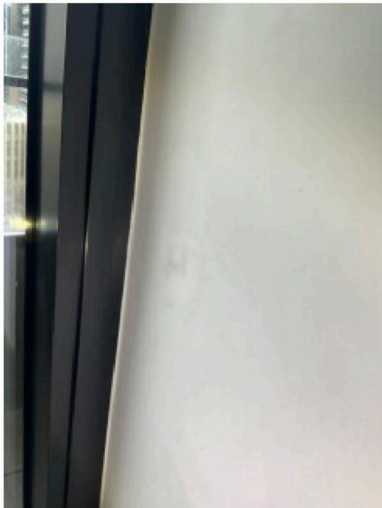
A patched section of the wall was observed. The repair appears visible and may indicate previous damage or repair work.
