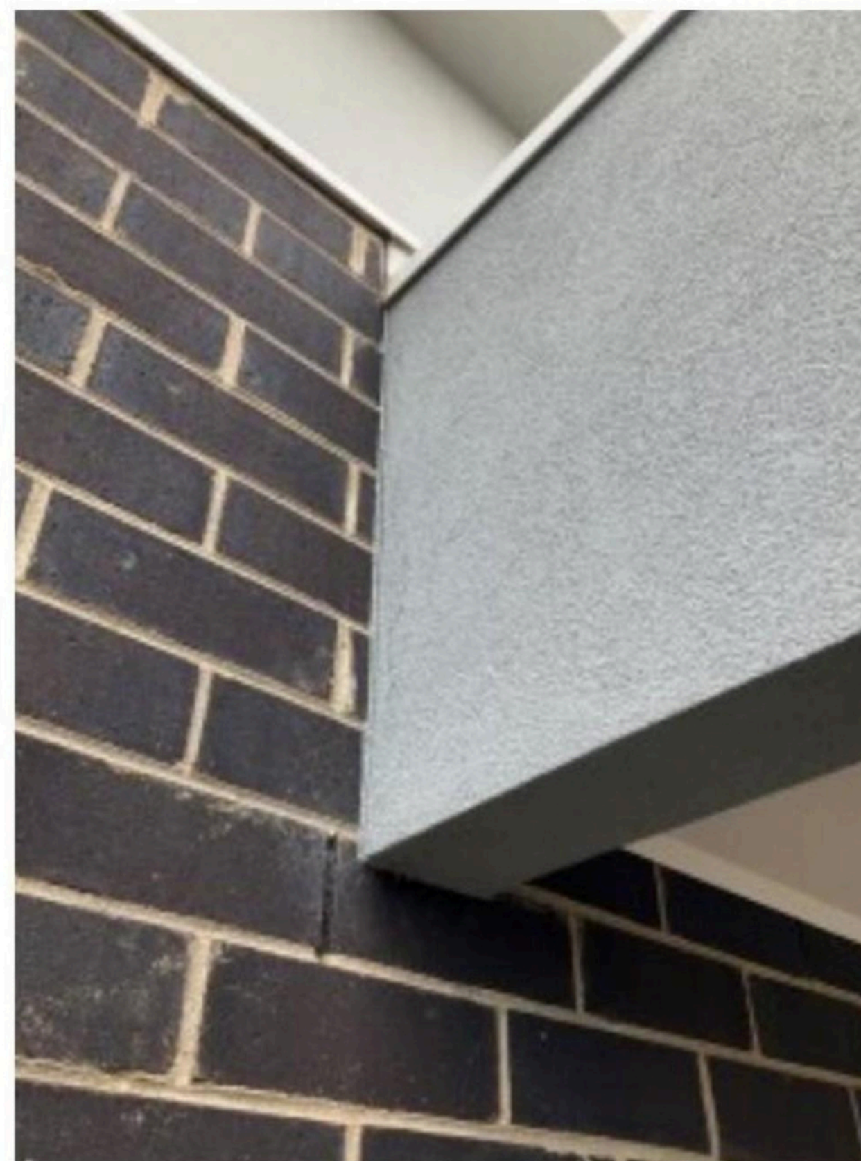
The exterior surface displays a noticeable crack where the rendered wall meets the brickwork. This separation indicates potential movement or settling issues that may require attention to prevent water ingress or further damage. Monitoring for any progression and repair would be advisable to maintain the integrity of the structure.
