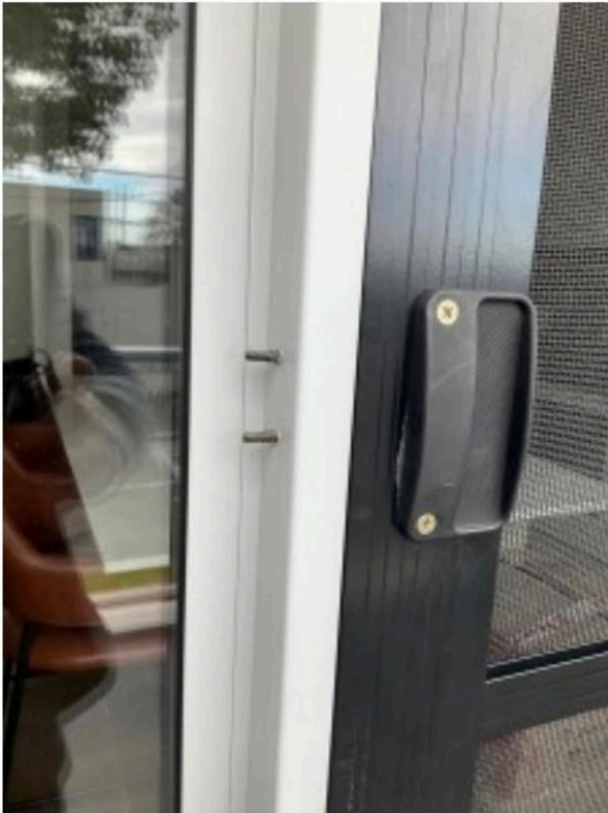
Incorrect screws used for sliding door installation. Handyman to rectify.
