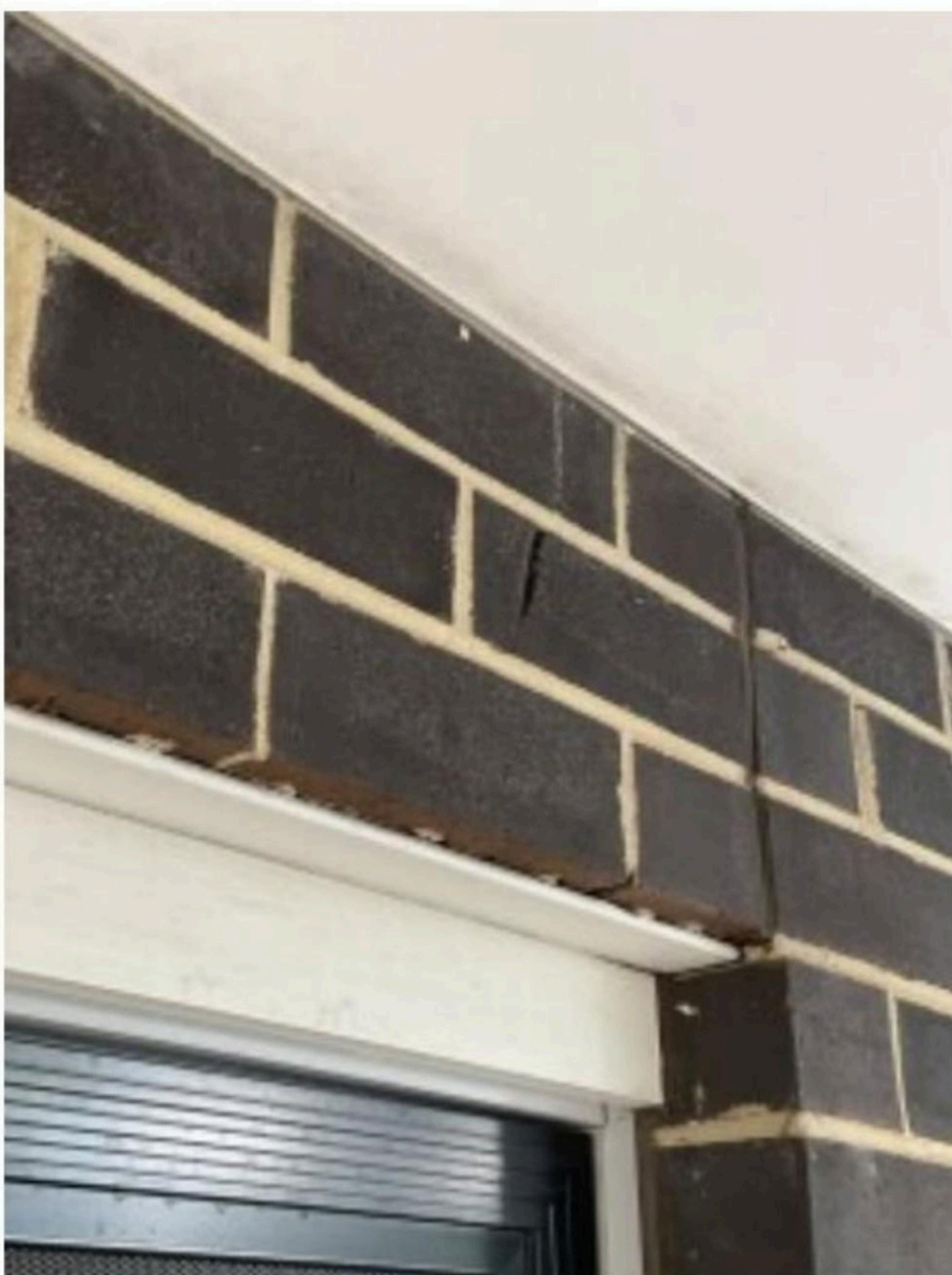
There is a crack in one of the bricks above the window. Repair or replacement is recommended to prevent water penetration.
